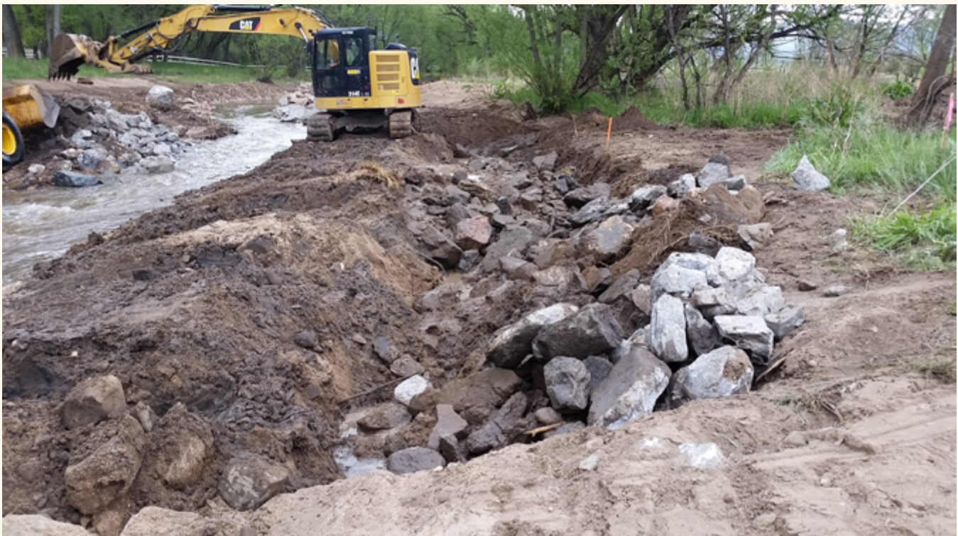
Setback riprap is buried away from channel bank | Photo courtesy of Colorado Water Conservation Board
