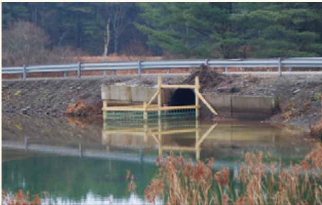
A flow device excludes beavers from a culvert and maintains flow of water | Photo courtesy of Skip Lisle, Beaver Deceivers International
