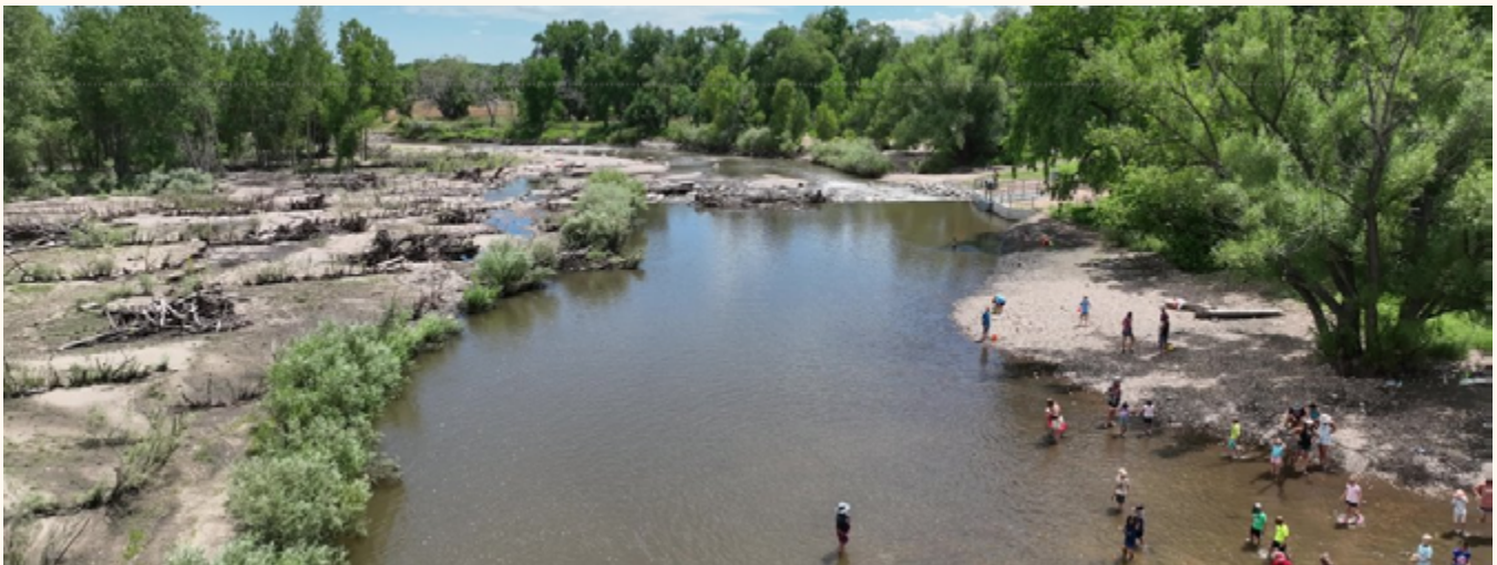
Large wood habitat features installed during restoration for habitat, infrastructure protection, and to support sediment transport processes | Photo courtesy of the City of Fort Collins
