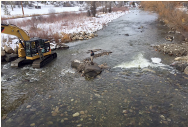
Excavators build a boulder structure where wood structures are not possible | Photo by Peter Van De Carr
