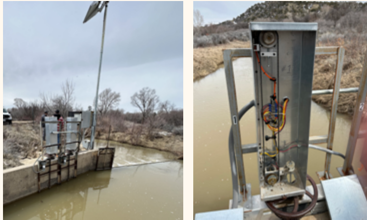
Installed automation control | Photo by Eric Peterson, Bureau of Reclamation
