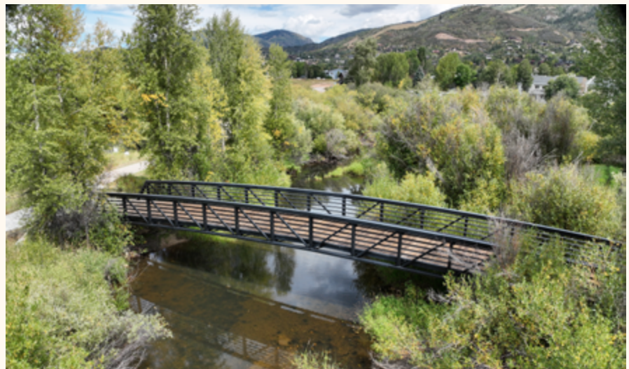
A widespan crossing doesn't have pillars to obstruct the stream | Photo by Roddy Beall, Zenobia Consultants
