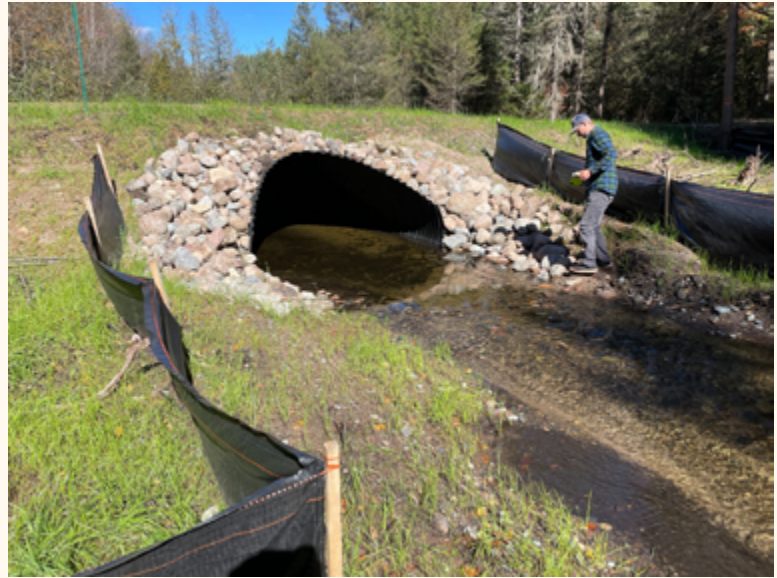
This “bottomless” pipe arch culvert maintains natural stream bottom conditions | Photo by Trout Unlimited
