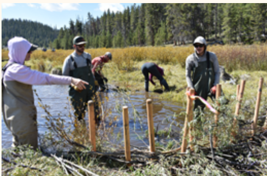
A post-assisted log structure detains water in the channel | Photo by Eli Smith, National Forest Foundation
