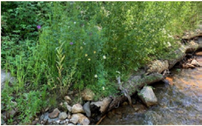
Willow toe, eight months after installation Photo from the Colorado Stream Corridor Construction Manual
