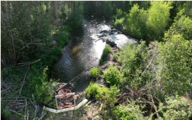
A permanent rock rundown diversion structure doesn't require annual excavation work | Photo by Roddy Beall, Zenobia Consultants
