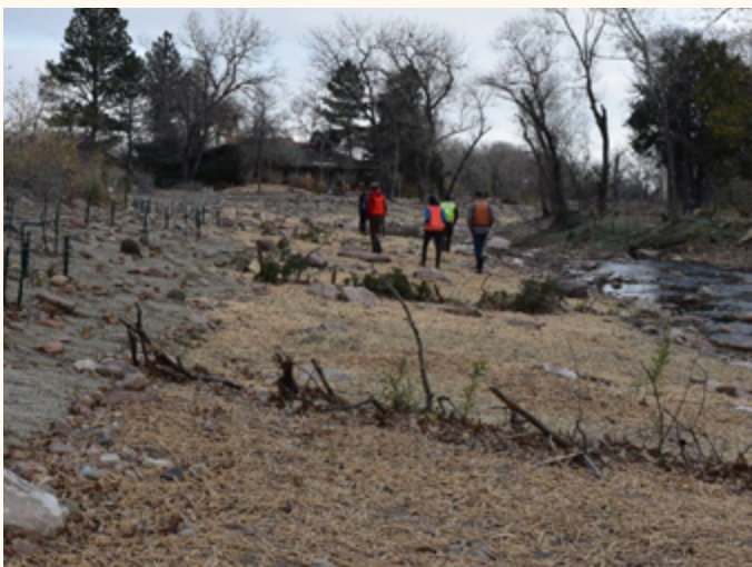
Brush trenches installed on a hydrologically connected floodplain Photo from the Colorado Stream Corridor Construction Manual
